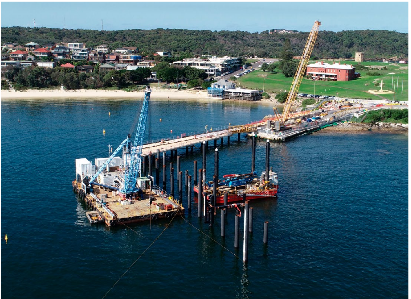
Kamay Ferry Terminals project, New South Wales. The project was recently completed by McConnell Dowell.
