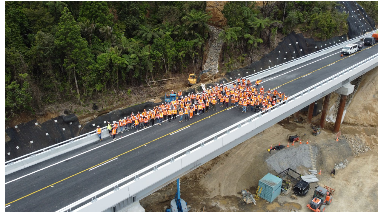
State Highway 25A Taparahi Slip Remediation, New Zealand Awarded 'Bridge Project Team of the Year' – New Civil Engineering Awards, London
