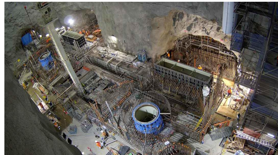
Kidston Pumped Storage Hydro, Queensland Expected productivities not achieved due to technical complexity
