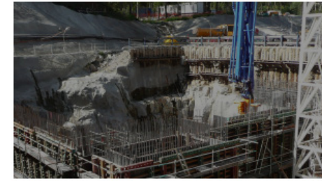
Hydropower and Dams
