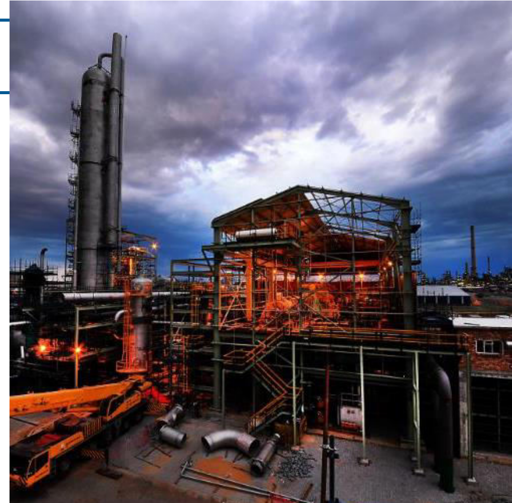
Aveng Grinaker-LTA M&E Nitric Acid Plant, Sasolburg
