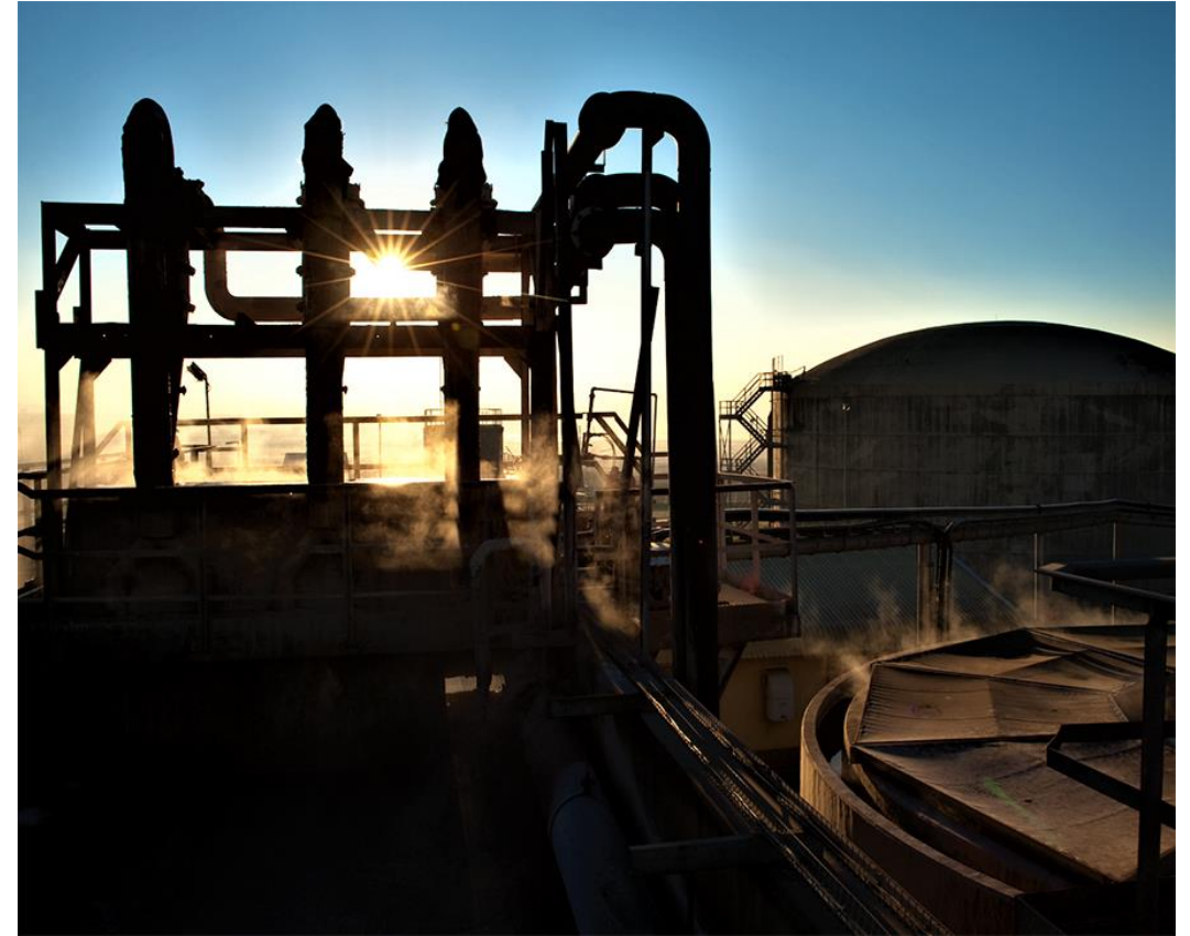
Aveng Water eMalahleni Reclamation Plant
