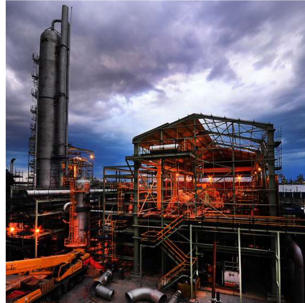
Aveng Grinaker-LTA M&E Nitric Acid Plant, Sasolburg
