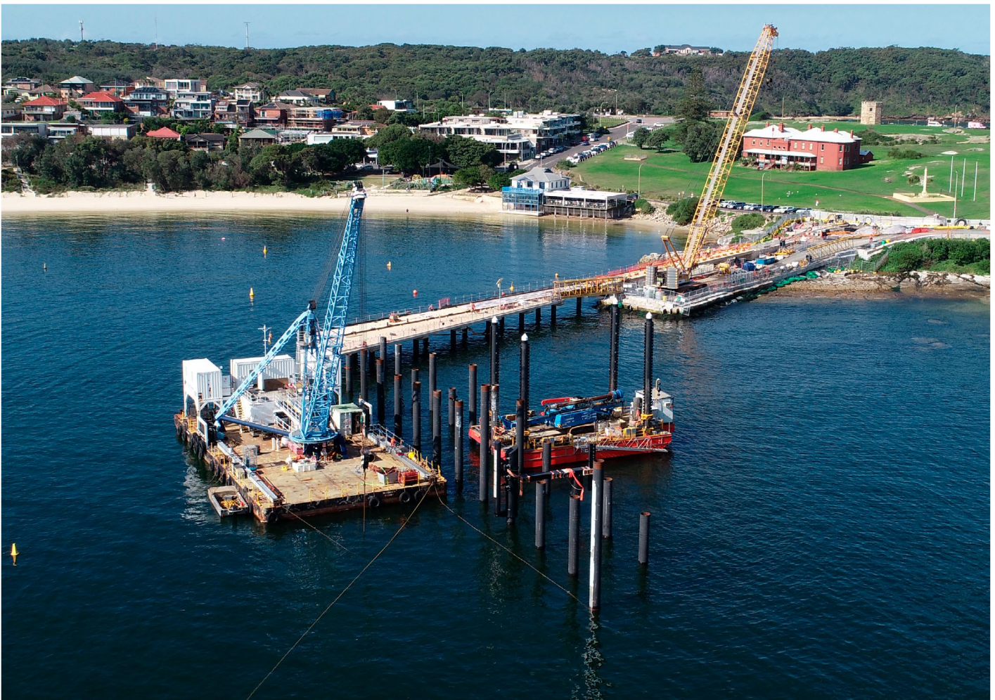
Kamay Ferry Terminals project, New South Wales. The project was recently completed by McConnell Dowell.
