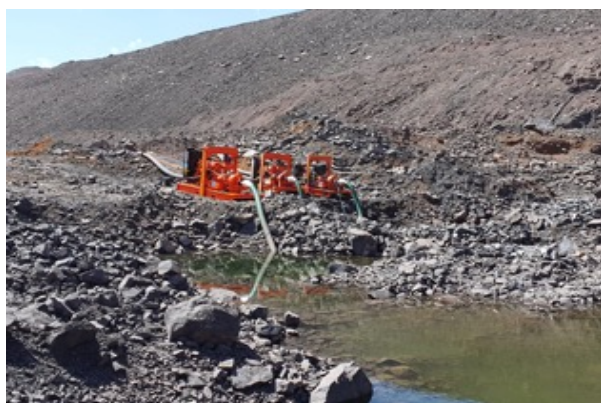
Pumping water from the pit into a storage dam, and then into water bowsers
