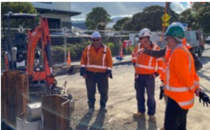
New Zealand general manager completing a safety leadership visit at Barber Grove Project, Wellington.
