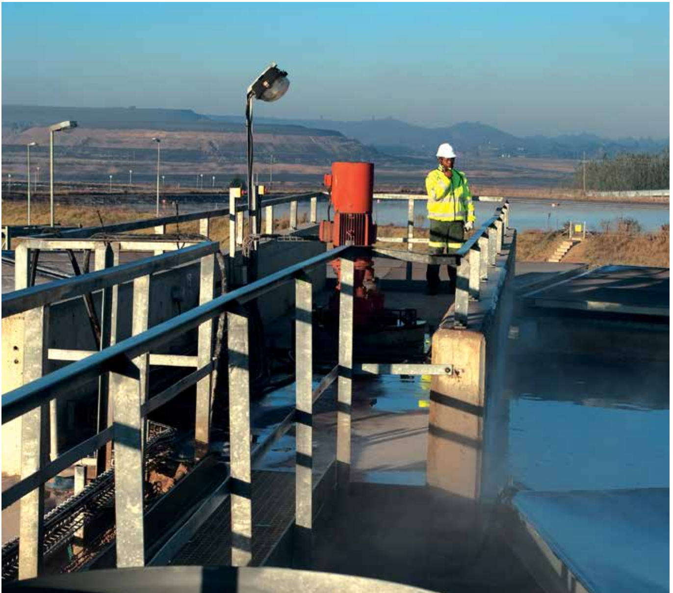
Water treatment plant, eMalahleni Project, Mpumalanga
